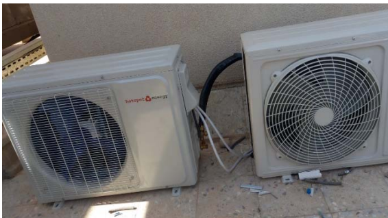
Fig.8: DC & AC air conditioner
