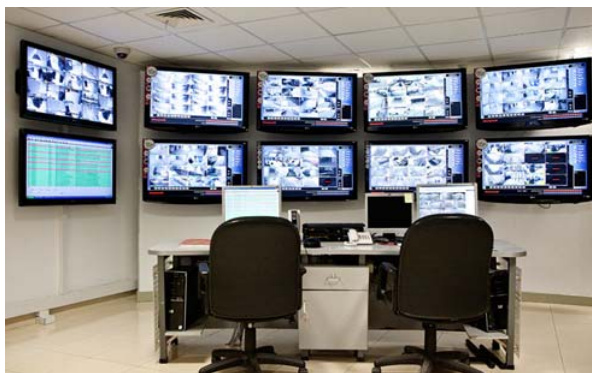
Fig. 4 - Alarm receiving centre [9]
