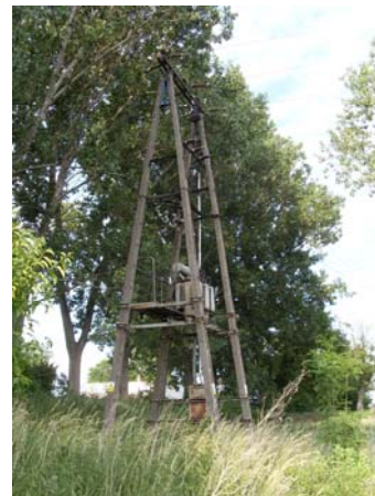
Fig 2. Overhead transformer station: STS – 20/250 type
