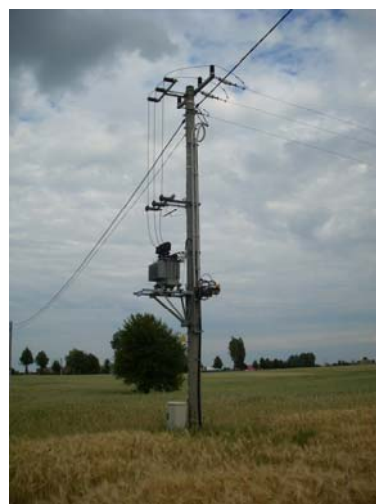
Fig 3. Overhead transformer station: STN type
