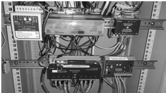
Fig.9. Cabinet with the TELETASK system modules used to control the temperature
