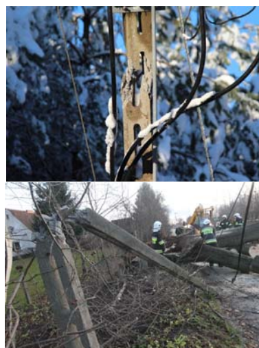
Fig.1. The examples of damages to overhead lines: the ageing of the structure [15], and damages caused by branches of trees [16]
